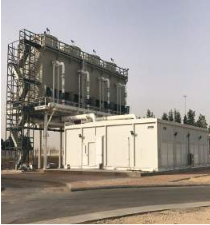
DCP CLIENT MEBCO - DAMMAM
