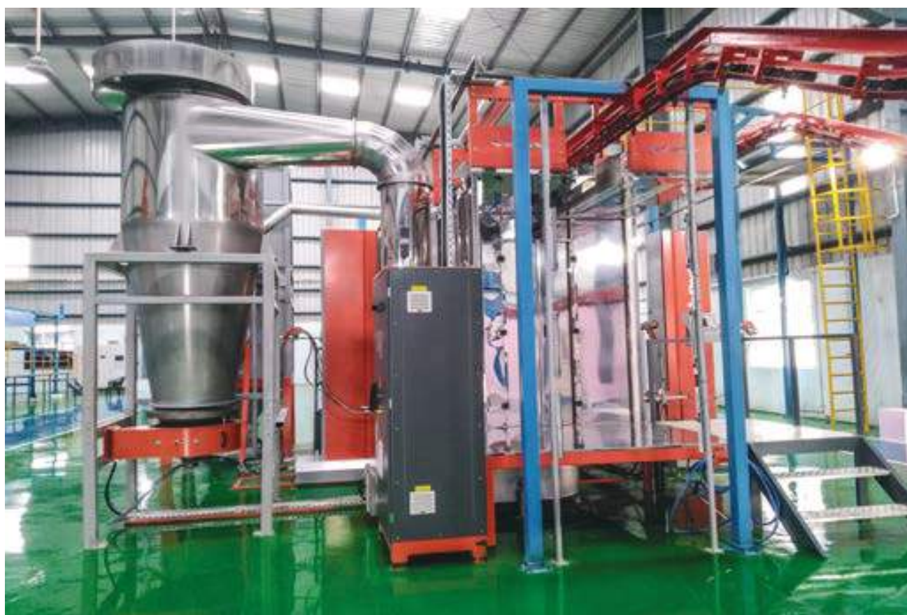
POWDER COATING STATION
