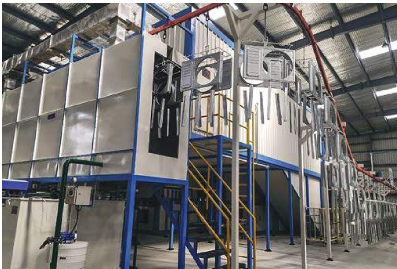
FULLY AUTOMATIC POWDER COATING PLANT FOR AIR CONDITIONER
